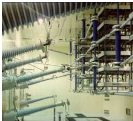
Figure 8: Suspended valve tower with polymer housed valve protection arresters (LADWP, California/USA, \pm 500 kV dc)
