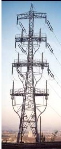
Figure 6 : 161-kV-tower with 6 cable terminations, protected by suspended polymer housed surge arresters (IEC, Israel)
